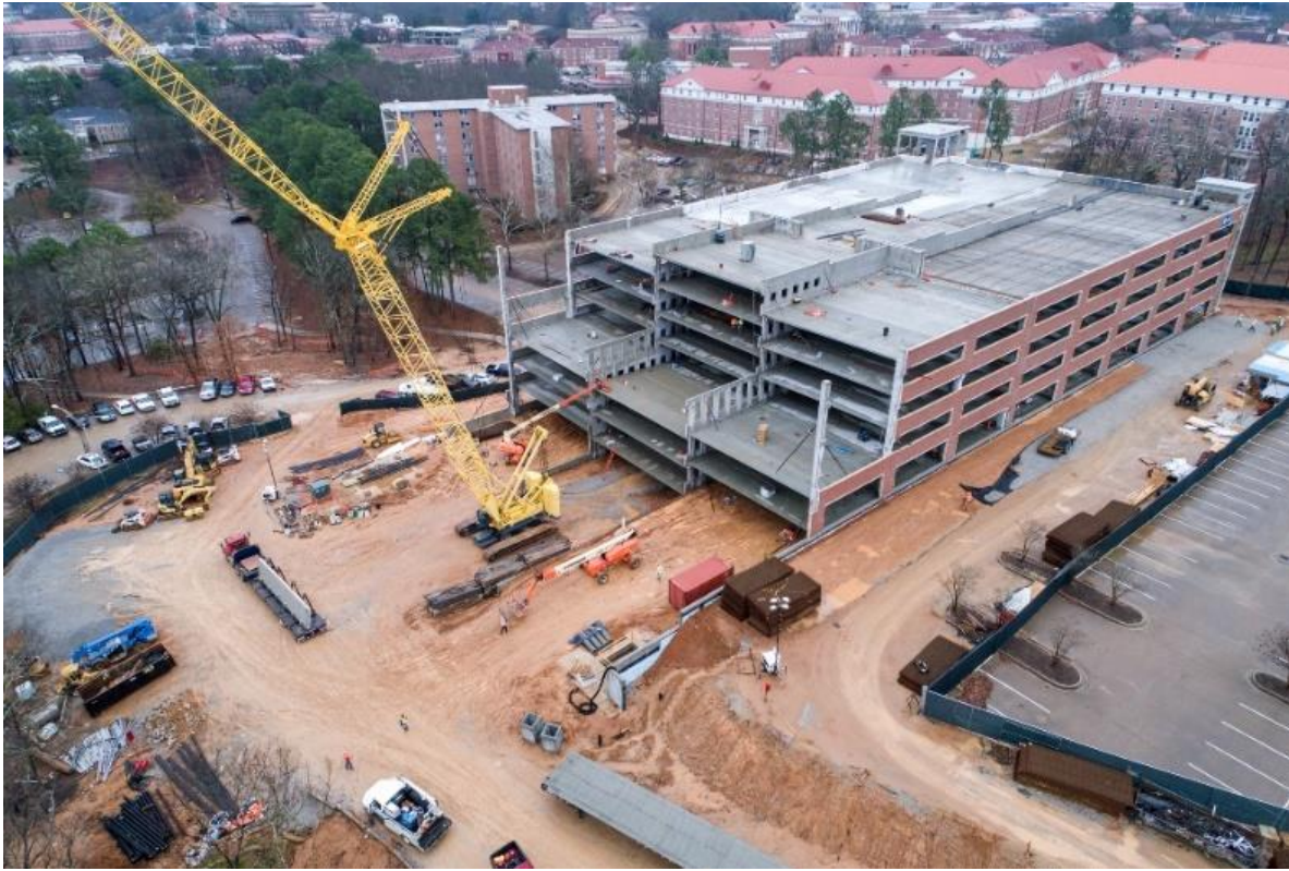
The crane in the central bay of the structure lifts precast pieces off trucks for placement.
