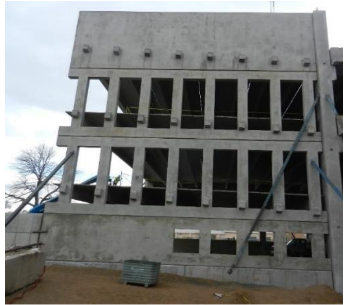
Photo 3 – Partially erected precast parking structure. Lite wall pieces, columns, inverted tee beams, and double tee beams are present. Temporary bracing stabilizes the structure until all pieces are in place and connected.
