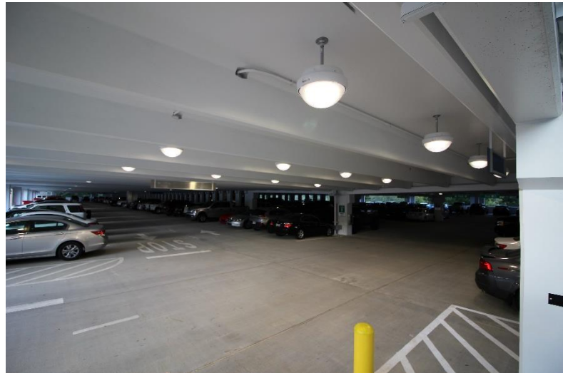
Photo 5 – A typical interior view of a precast parking structure with a 12'-0" floor-to-floor height and stained ceilings.
